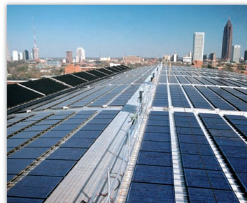
(c) Roof-top solar array
