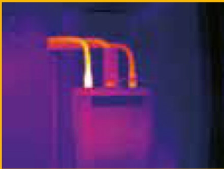
Poor connection and internal damage
