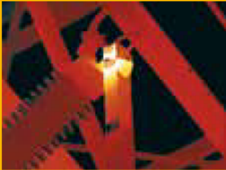
Incorrectly secured connection
