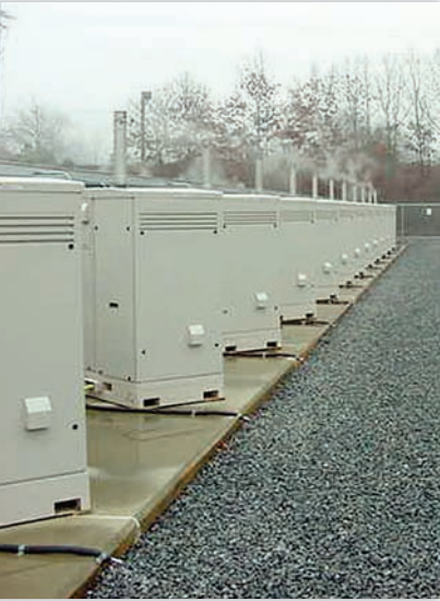
◀ FIGURE 13.37 The Long Island Power Authority has installed 75 stationary fuel cells to provide reliable backup power.
