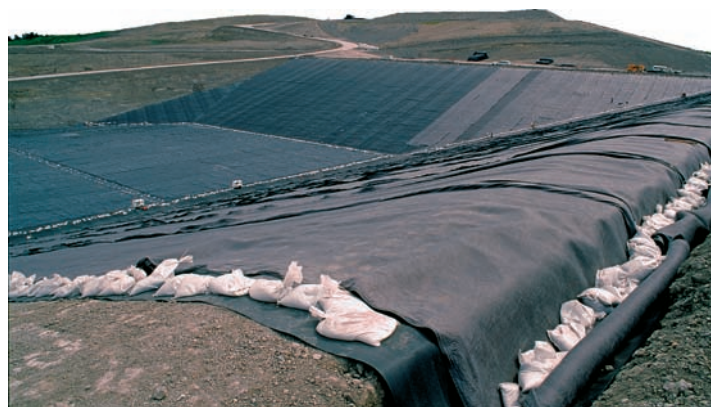
▲ FIGURE 14.6 A plastic liner being installed in a sanitary landfill. This liner and a bentonite clay layer below it prevent leakage to groundwater. Trash is also compacted and covered with earth fill every day.
