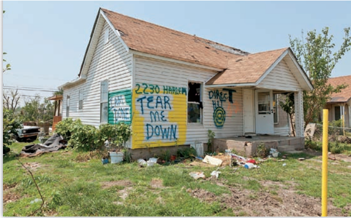
▲ FIGURE 15.10 Many old, industrial cities in America's "rust belt" are tearing down tens of thousands of abandoned, derelict houses. This opens up an opportunity for redevelopment with gardens, green belts, diverse flexible housing, walkable neighborhoods, and other features of smart growth.
