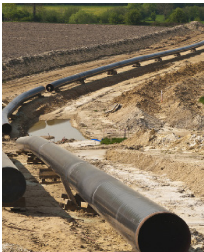
Natural gas transmission lines
