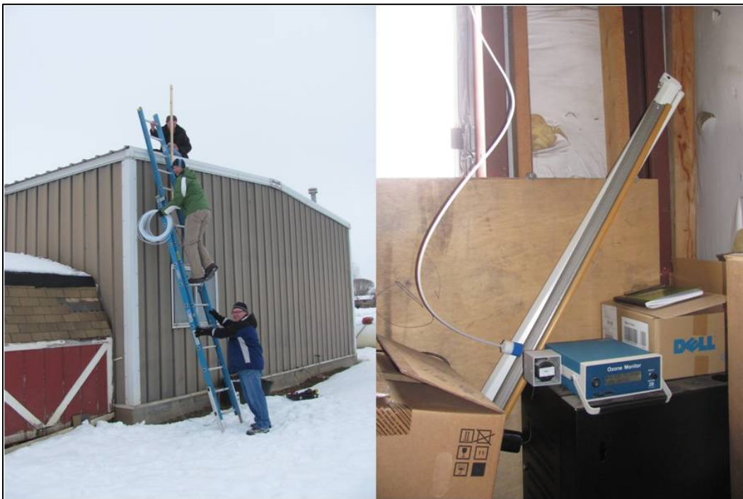
Figure 3-1. Installation of the sample line and 2B Ozone Monitor at the Roosevelt location.
